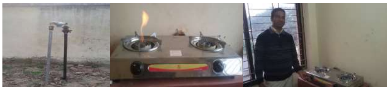
Fig 2: Gas line connection in Regional station
